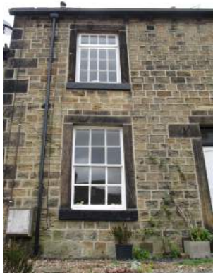
Plate 29: 6 over 6 sash window (bottom) on No. 12 Darton Road. The top window has been replaced
