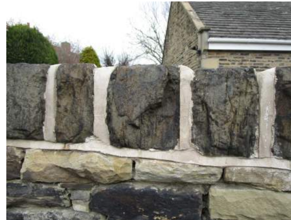
Plate 51: Ribbon and cement pointing detract from historic walling and is a cause of erosion
