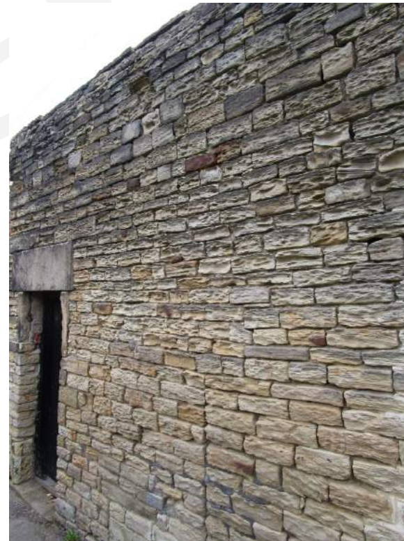
Plate 24: Sandstone outbuildings, rear of Victoria Cottage Institute, Darton Road - where cement pointing has been used in the past, the face of the stonework has eroded
